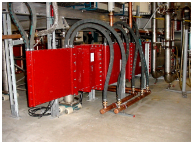
400-kW-Ferrit-Absorber am Sender HERA-WR
